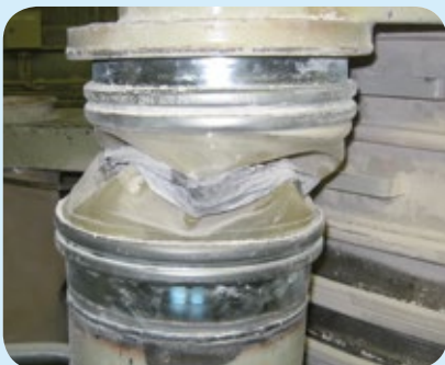
— Installation zu eng
